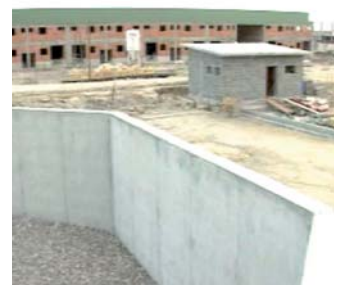
Diesel tank bund
