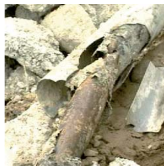
Corroded steel pipe
