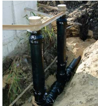
6" double wall elbow and tee in close proximity
