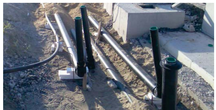
4" double wall pipe risers in foreground next to road tanker pad prior to backfilling
