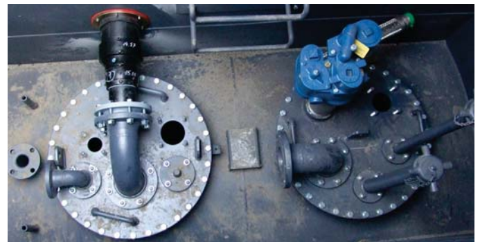
IST Submersible Turbine Pump mounted on fuel tank manway cover awaits connection
