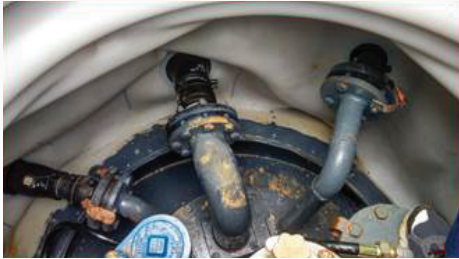
Tank chamber failure
