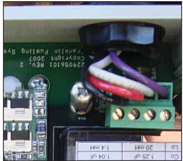
Figure 12: Wiring Connection to DTU
