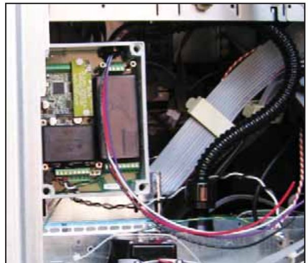
Figure 13: Wires in Flexible Conduit
