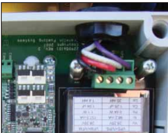
Figure 16: Terminal Block Wiring
