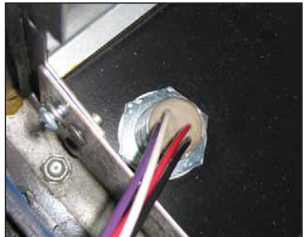
Figure 5: Potted Nipple Installed
