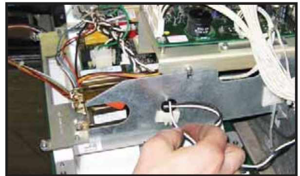
Figure 9: Power Harness Wiring
