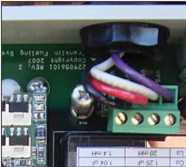
Figure 14: Wiring Connection to DTU
