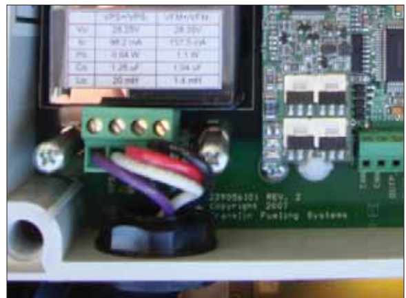
Figure 13: Wires attached to DTU
