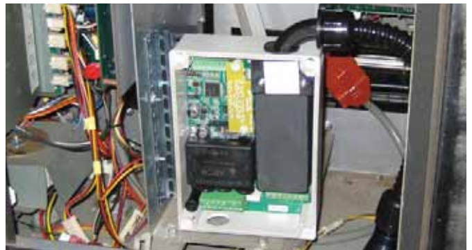
Figure 13: Reinstall Barrier Cover
