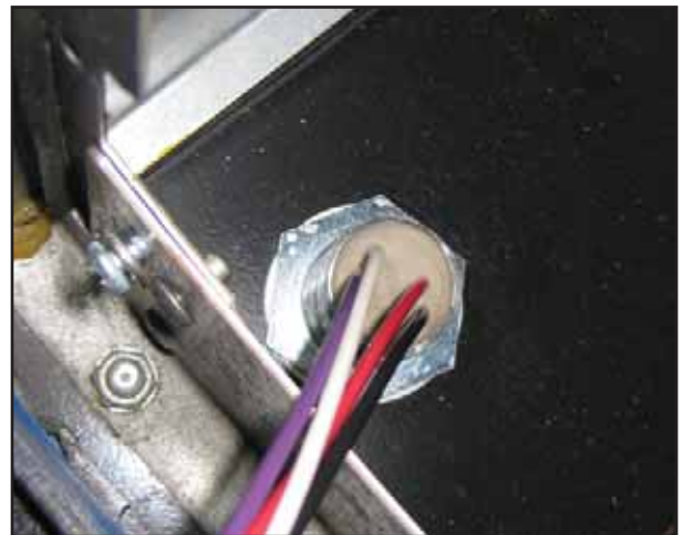
Figure 4: Potted Nipple Installed
