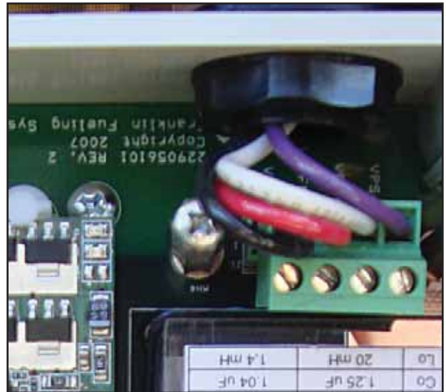
Figure 14: Wiring Connection to DTU
