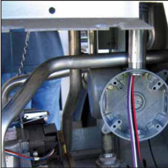
Figure 8: Junction Box Connected to Potted Nipple
