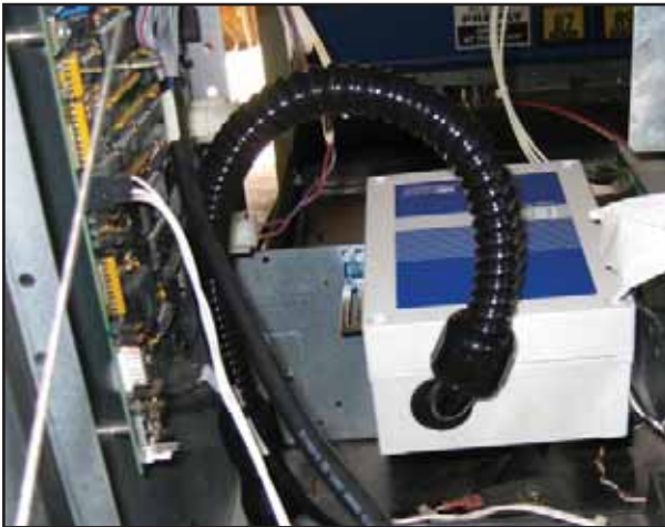
Figure 16: DTU Installed with Cover On
