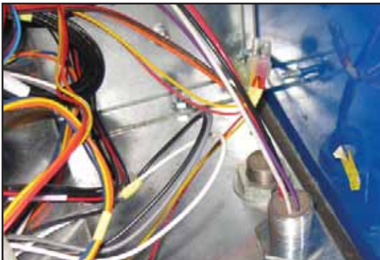
Figure 8: Potted Nipple Installed
