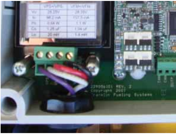
Figure 16: Wires Connected to DTU
