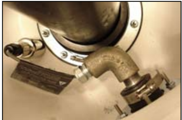
Sensor Installed in Fiberglass Secondary
