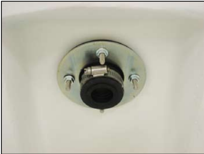
Figure 4: Inside view of FEB-075-D Installed
